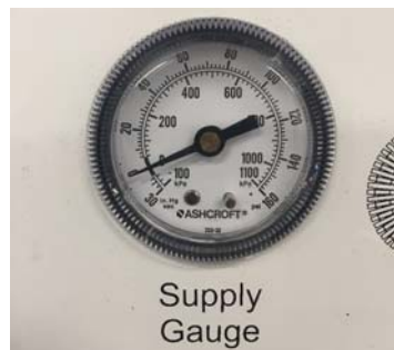
Figure 4-3 Setting the pressure on the Supply gauge (10-21 kPa)
