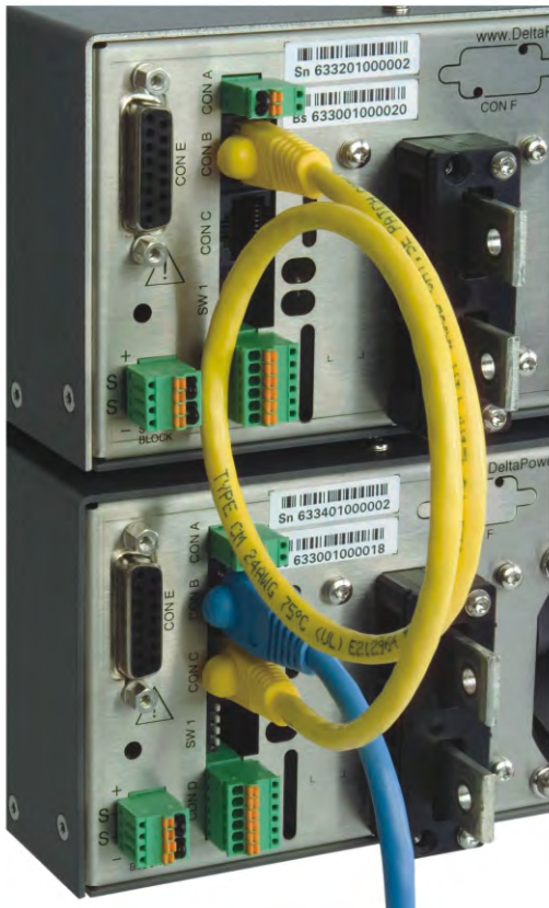
fig. 2 - 22 Use standard UTP cables (RJ45) for Master / Slave operation
